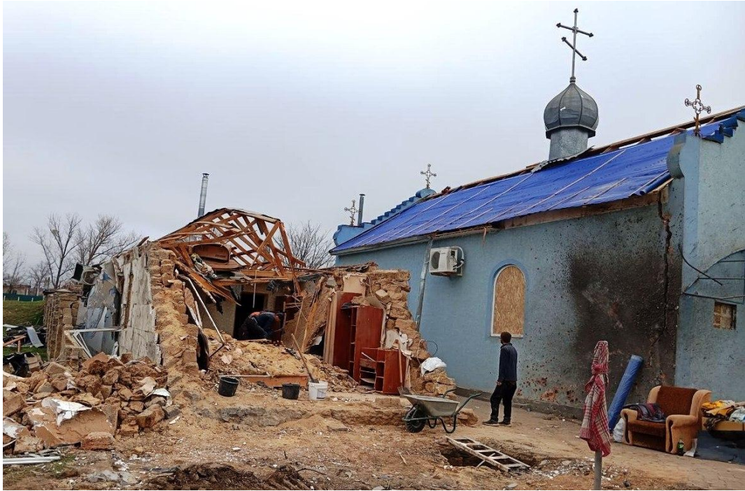
Orthodox Church – roof covered and window boarded up to stop the elements getting in, but the priest's house (left) is badly damaged
